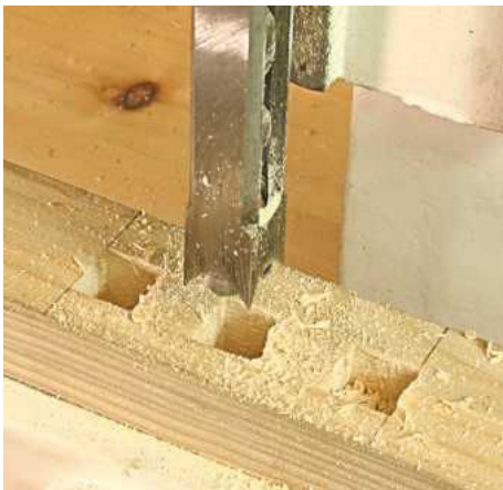
▲ Pic.8 Jeff was sure to follow the advice to cut each end before removing the remainder
